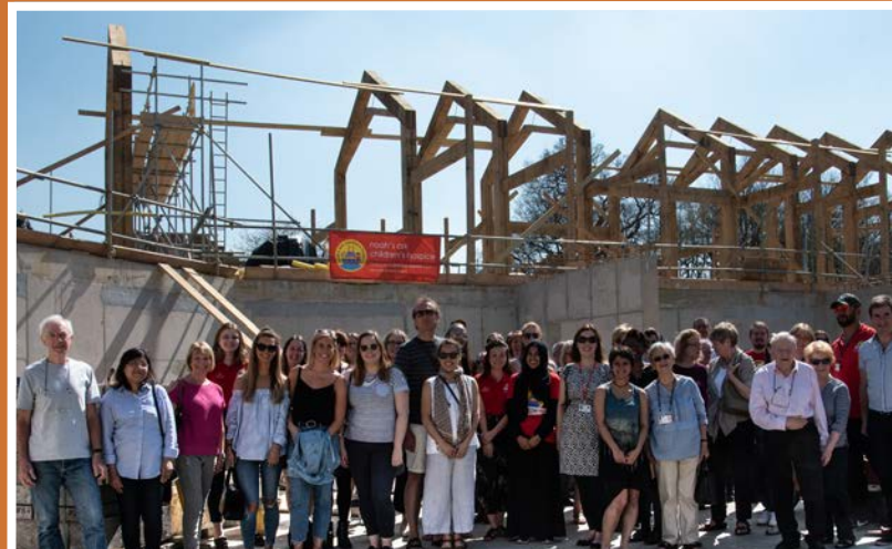
Residents and supporters gathered at the Noah's Ark construction site to celebrate the topping out of the atrium for the new children's hospice
