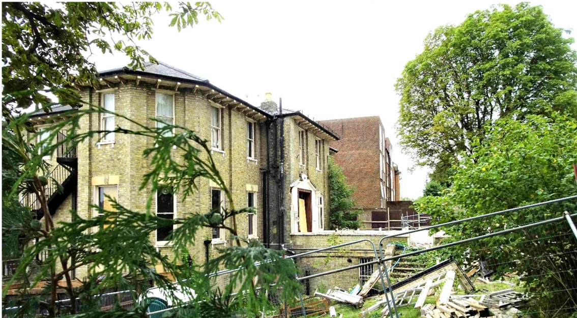
33 Lyonsdown Road – RIP the main entrance conservatory
